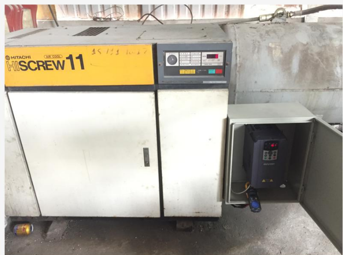
Inverter CT100-15KW controls screw air compressor
