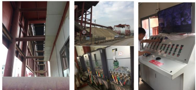
CT100 185KW for conveyor belt
