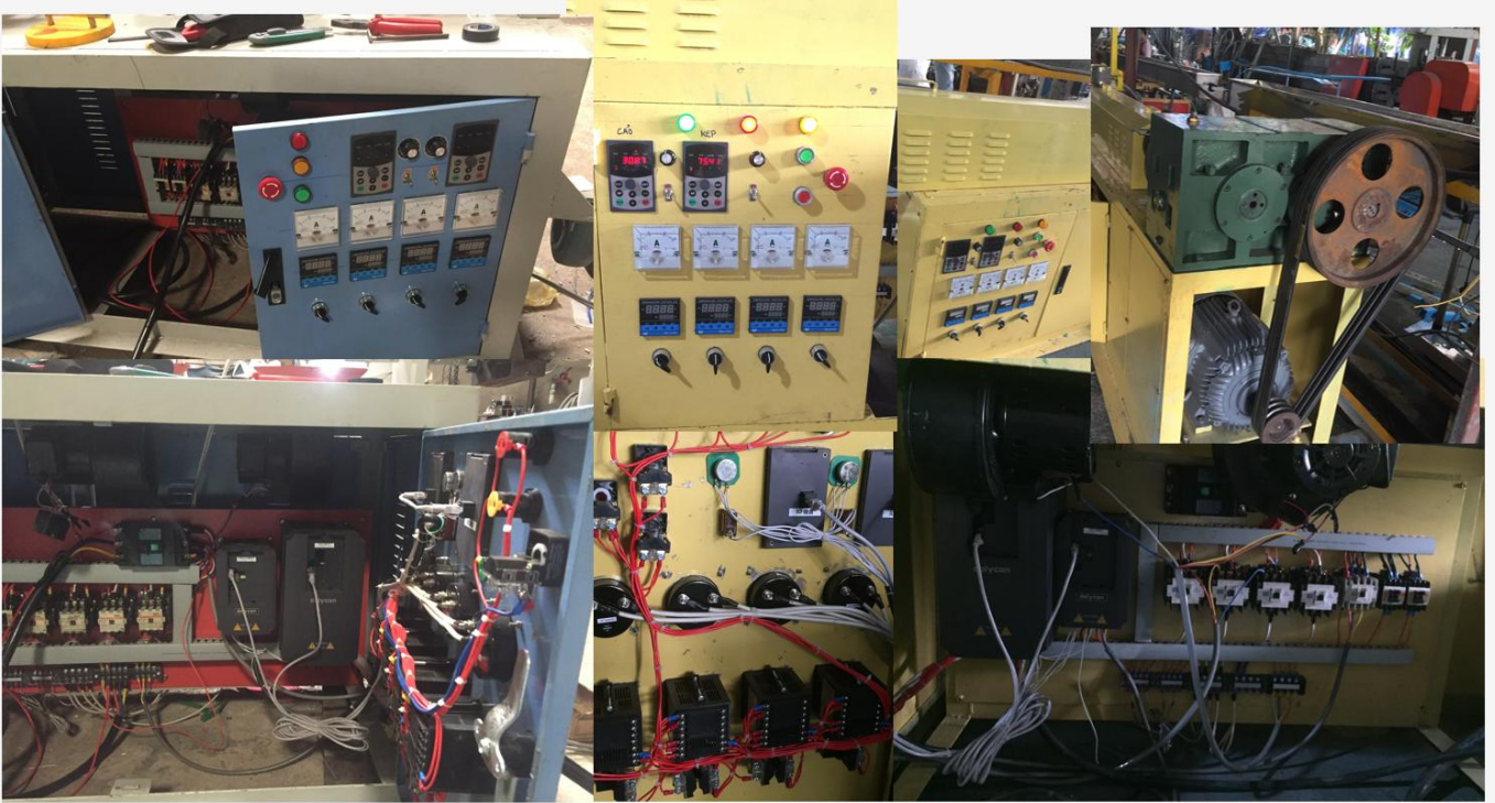
Inverter CT100 controls PE plastic forming machine
